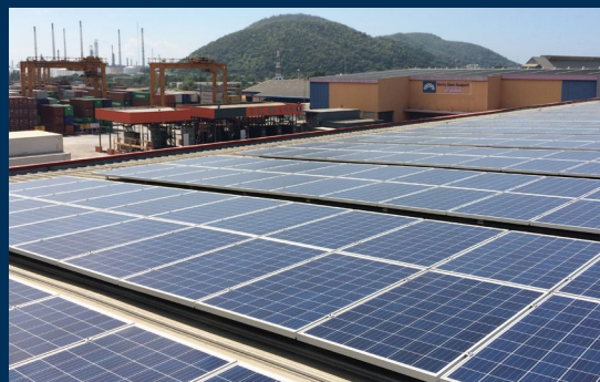
Location | Chonburi Facility | Warehouse
