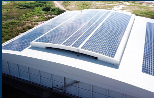
Location | Samut Sakhon Facility | Cold Storage
